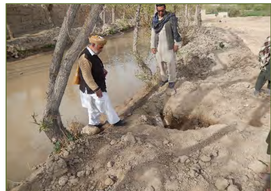
A view of selected site for protection wall along on Charamgar canal
